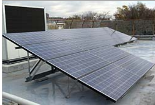
Photovoltaic panels installed on roof
