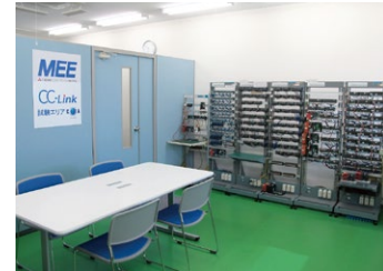
Conformance testing lab
