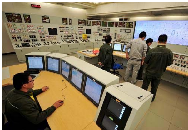
Central Monitoring Room
