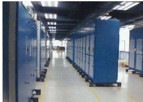
Digital Instrumentation and Control System
