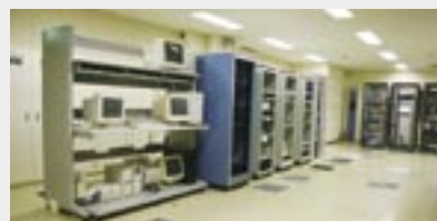
Computer Room Unnecessary computers were disposed of, new models with low power consumption installed, and the number of operating air conditioners reduced to cut power consumption by 70%. The required space was also reduced by two-thirds.
