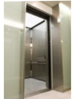
Barrier-free elevator (Head office building in Tokyo)
