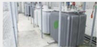
Transformers Transformers were updated with highly efficient models made by Mitsubishi Electric. Equipment will continue to be revamped as needed to make it possible to reduce energy consumption by 25% by 2010.
