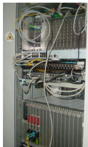
Fig. 2 GE-PON located in the central office
