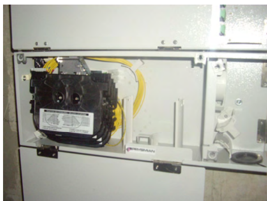
Fig. 1 Optical splitter located in the apartment basement
