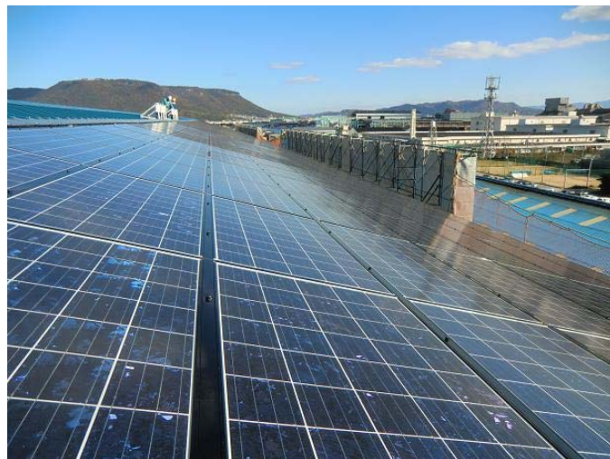
Mitsubishi Electric PV System installed on the roof of Makita's main factory
