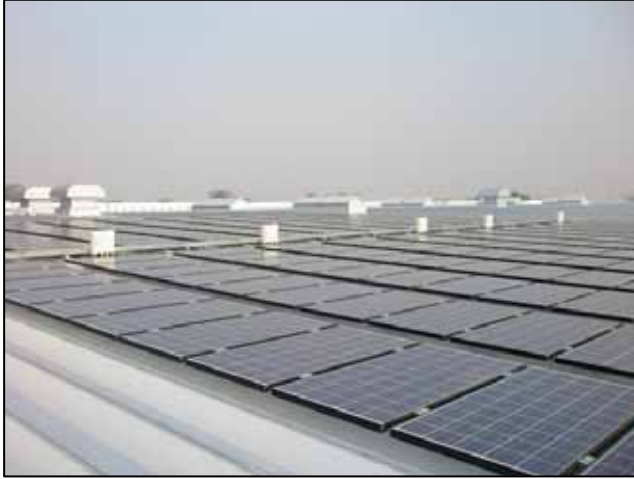
Fig. 1) 51 kW PV system on the warehouse roof (above)
