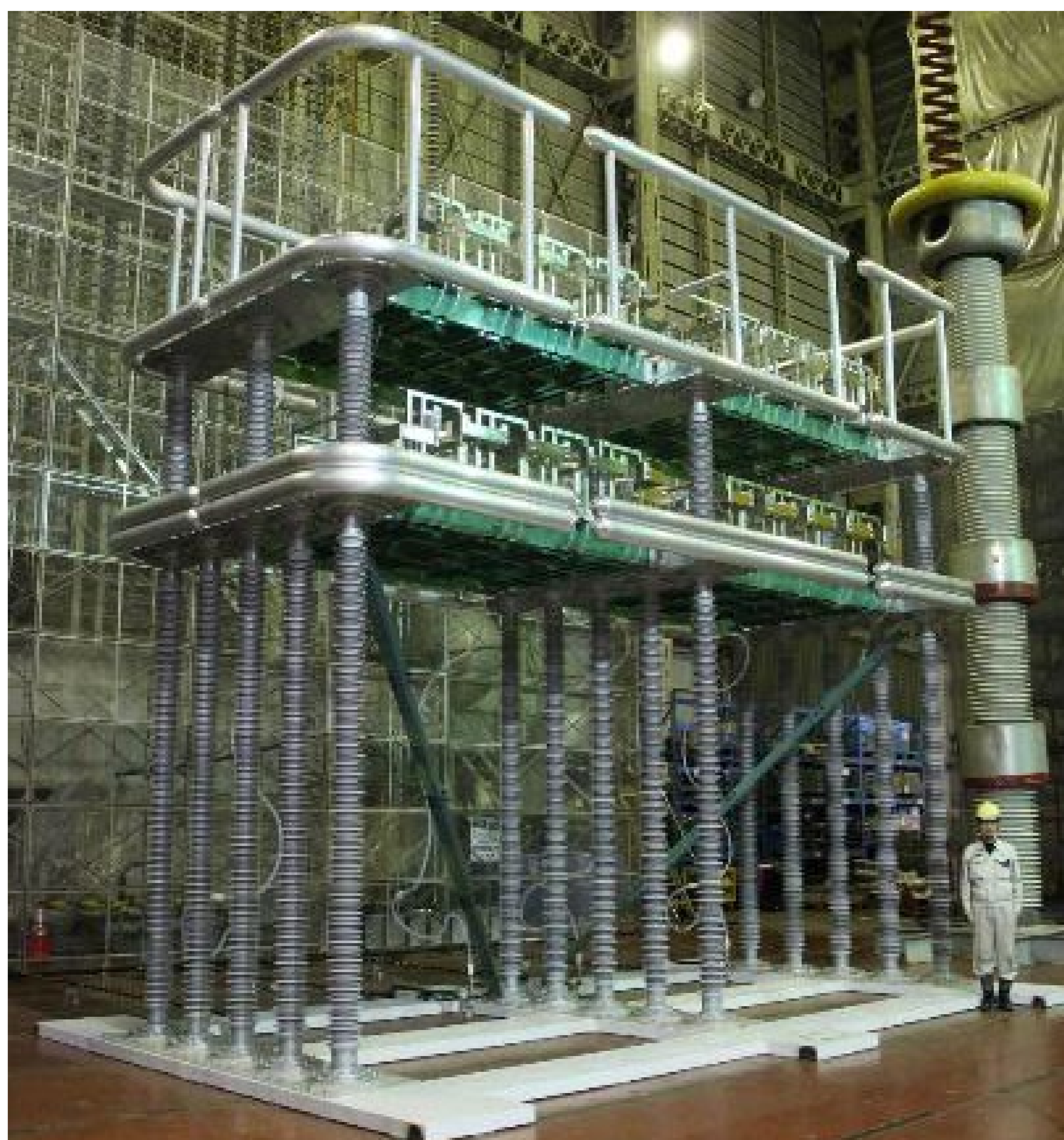
400 kV valve tower
