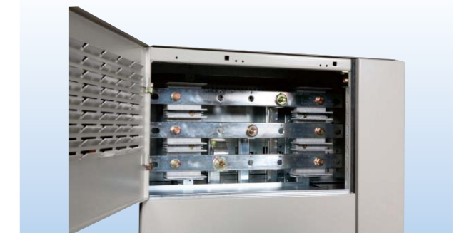
Horizontal busbar (rear view)
