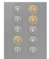
Car operating panel
