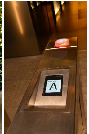
User’s assigned elevator displayed on security gate’s LCD indicator
