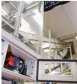
Production volume display device where C Controller has replaced PCs
