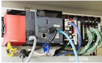
PLC on the back of the performance testing machine. The C Controller in the center has USB, LAN, and RGB interfaces like a PC
