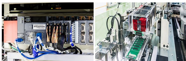
Base unit test equipment: one of the systems using the C Controller. The C Controller is used to control the test to check the input/output of the base unit and store test results in the production control database
