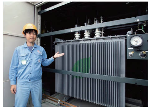
10 transformers installed in enclosures on the roof of the E1 Building (three-phase 750kVA x 3, three-phase 500kVA x 1, single-phase 300kVA x 4, single-phase 200kVA x 1) (Right: Transformer inside an enclosure)
